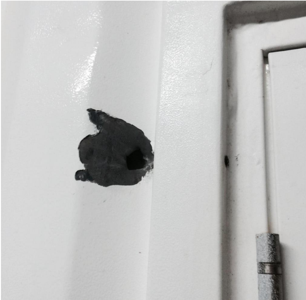
A bullet hole in a wall at Manus Island Immigration Detention Central following an incident between February 16 and 18, 2014. Image supplied 1 May 2014. © AAP Image/Supplied
