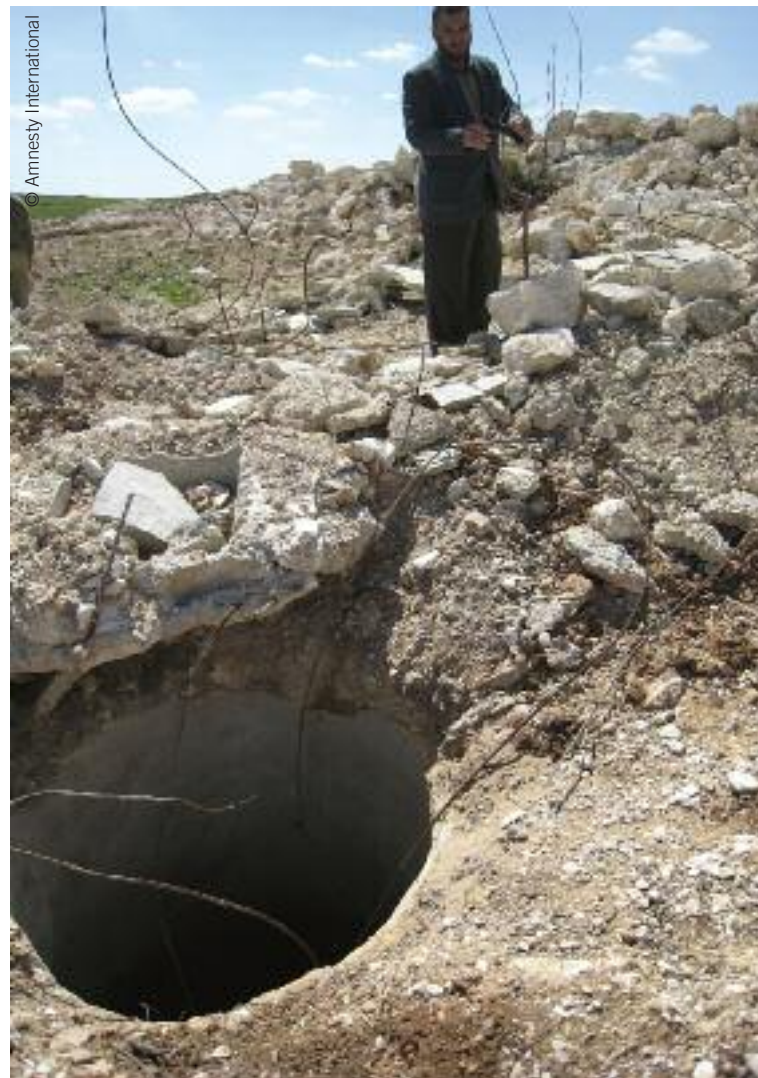
Above: Destroyed water cisterns in Beit Ula, March 2008. Below: A water tank in the West Bank village of 'Aqaba, May 2008.
