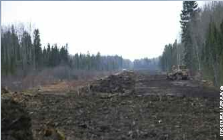
inset: A massive natural gas pipeline under construction in Lubicon Cree territory, licensed by the provincial government despite an unresolved land dispute. Alberta, Canada.
