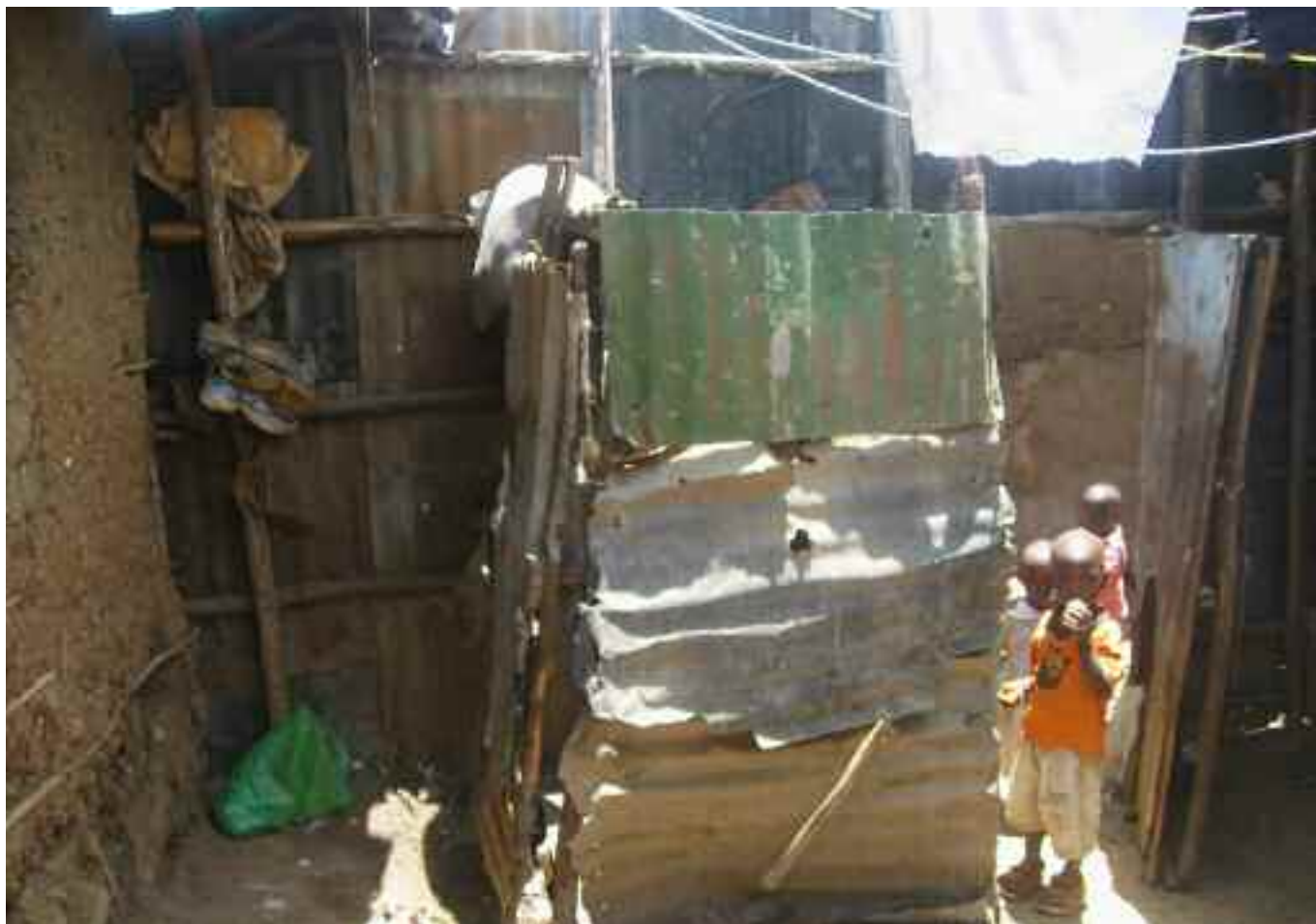
A private bathroom in a plot in Korogocho, Nairobi, shared by approximately 10 families living within the plot.
