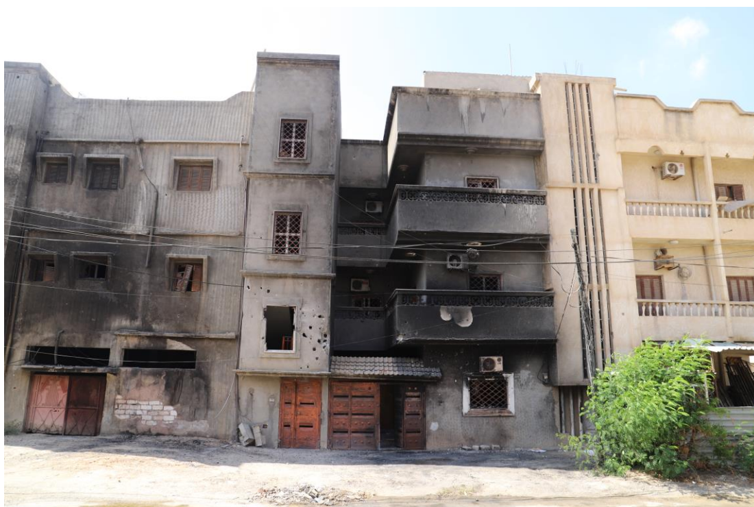
A building in Qasr Bin Ghashir damaged by a GNA artillery strike which killed at least five civilians and injured more than a dozen residents and bystanders in and around the building on 14 May 2019. ©Amnesty International
