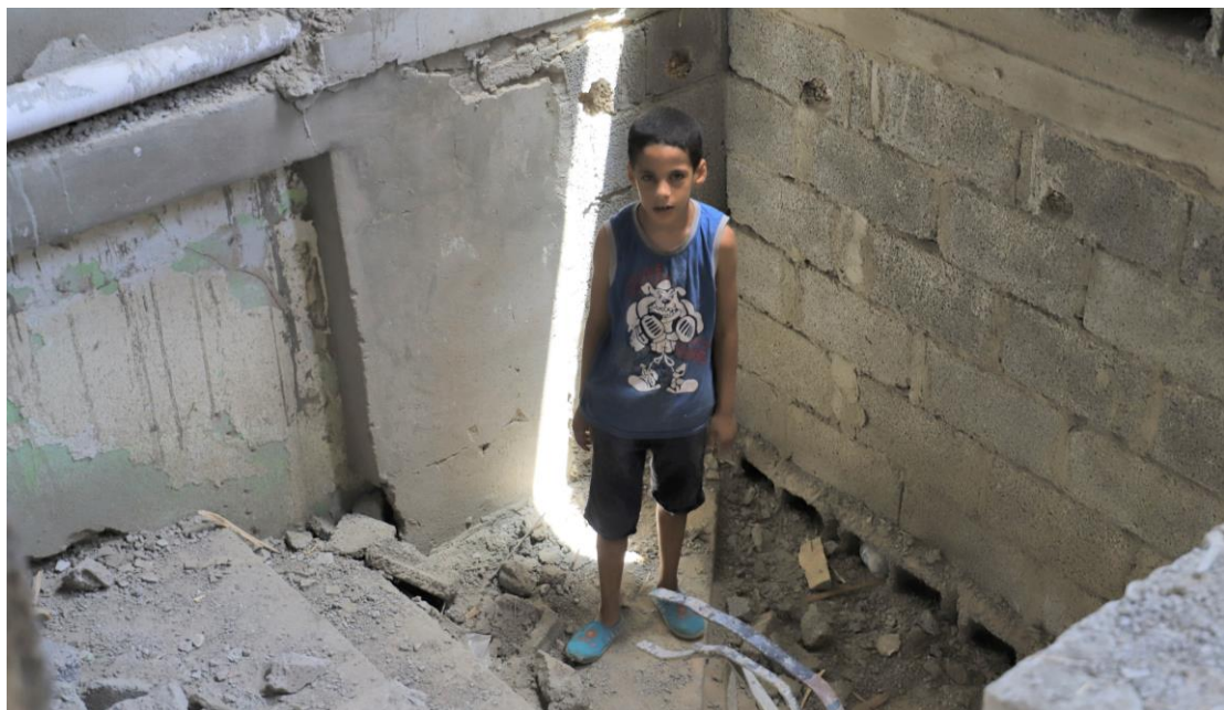
A child in his home damaged by a Grad rockets fired by the LNA into the Abu Salim neighbourhood of Tripoli, killing Nouredine Ahmad Ben Mansour on 16 April 2019. ©Amnesty International
