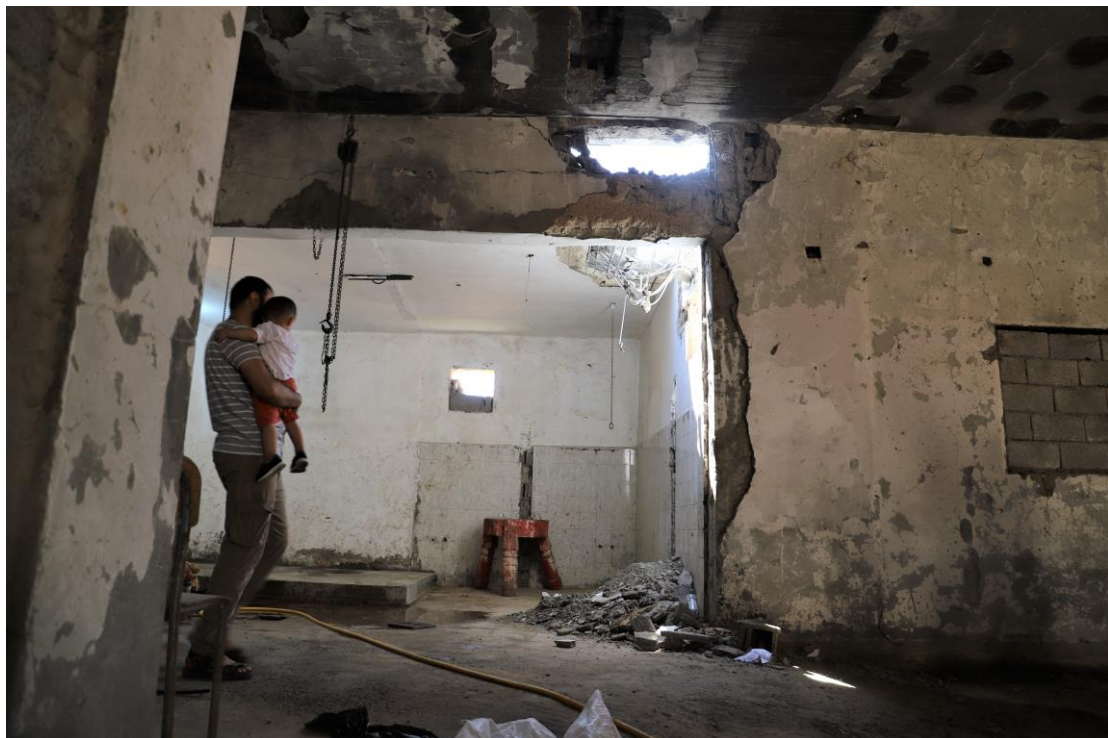
A house in the Souq al-Joumaa neighbourhood of Tripoli damaged by an artillery strike which injured three civilians on 11 August 2019. ©Amnesty International
