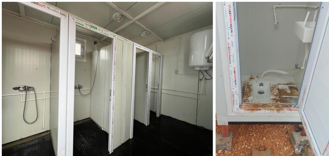
Inaccessible showers and latrines lacking ramp access, handles, ropes or chairs as observed by Amnesty International's researchers during their March 2023 visit to camps in four of the provinces that were most affected by the earthquakes. None of the 21 displacement sites visited by the researchers contained sanitation facilities that were accessible to persons with disabilities, a wider pattern confirmed by aid workers. © Amnesty International
