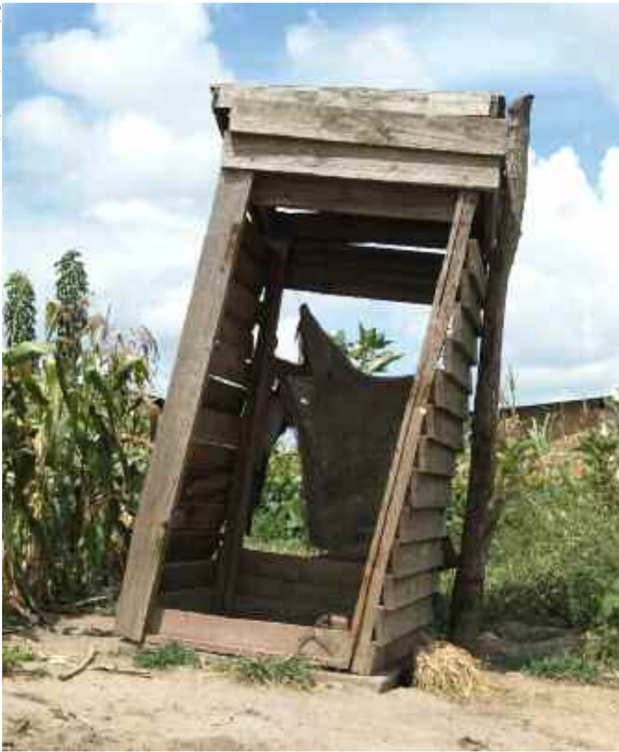
A toilet at Hopley. Thousands of people have lived for more than five years with little or no access to basic services such as water, sanitation, education and health care.
