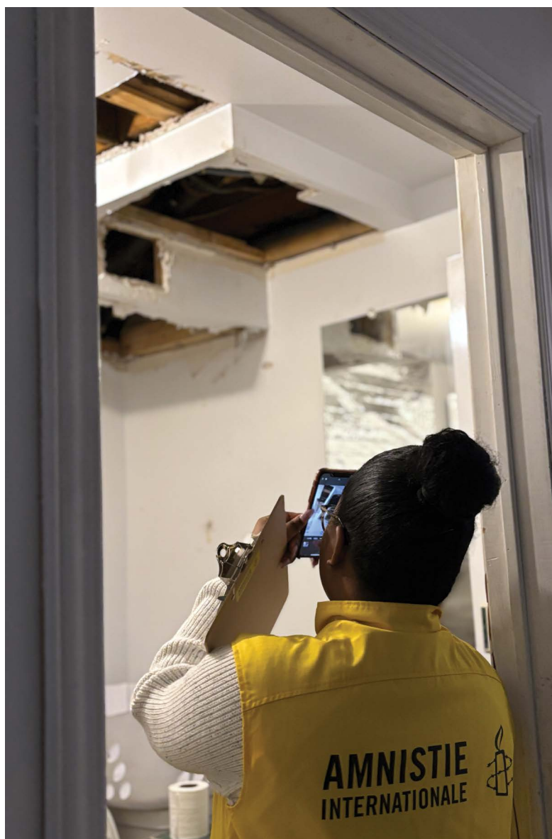
Hole in the ceiling of a Manawan's house
