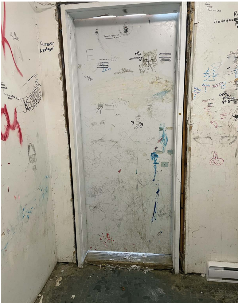
Leaky door in a residential building of Manawan
