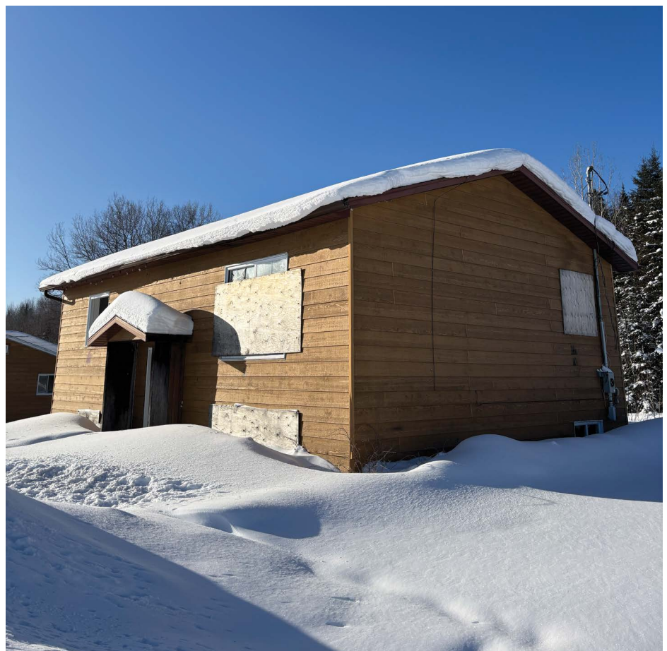
Condemned house in Manawan
