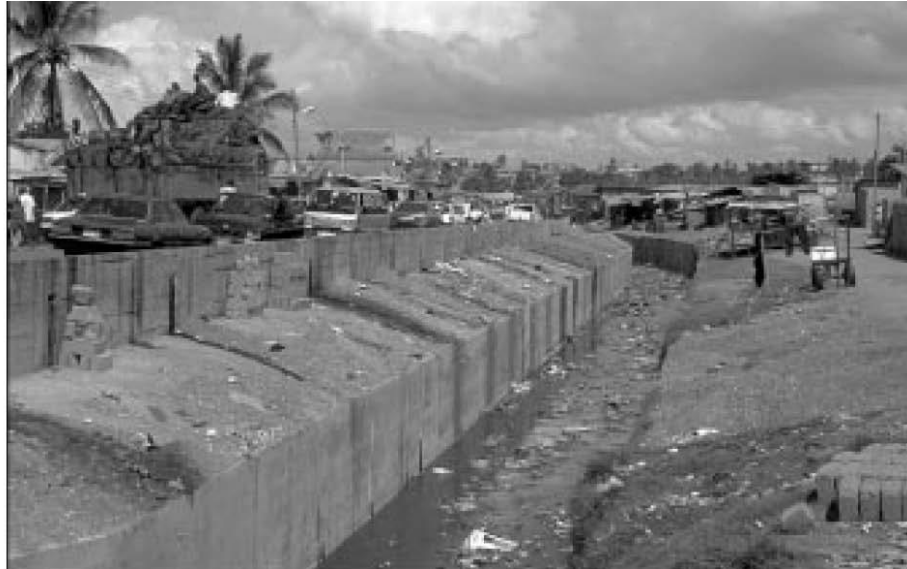
Sewerage and drainage is a major public health problem in cities in developing countries around the world. Here in Accra, Ghana, the sewers overflowed in 1995, leading to loss of life and destruction of property.
