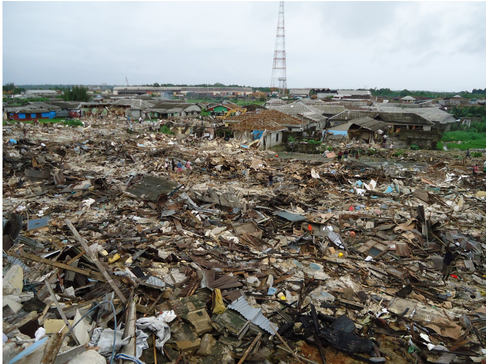
Hundreds of buildings destroyed as the demolitions continued on day 2, Thursday 28 June 2012.
