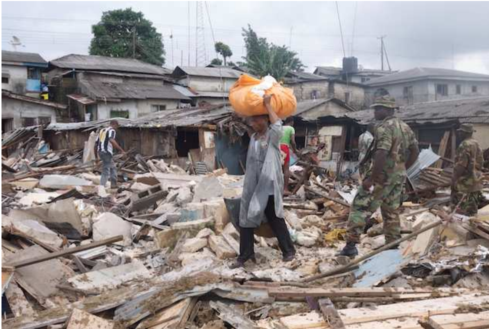
Security officers from the JTF supervising the Abonnema Wharf demolitions- Wednesday 27 June 2012.
