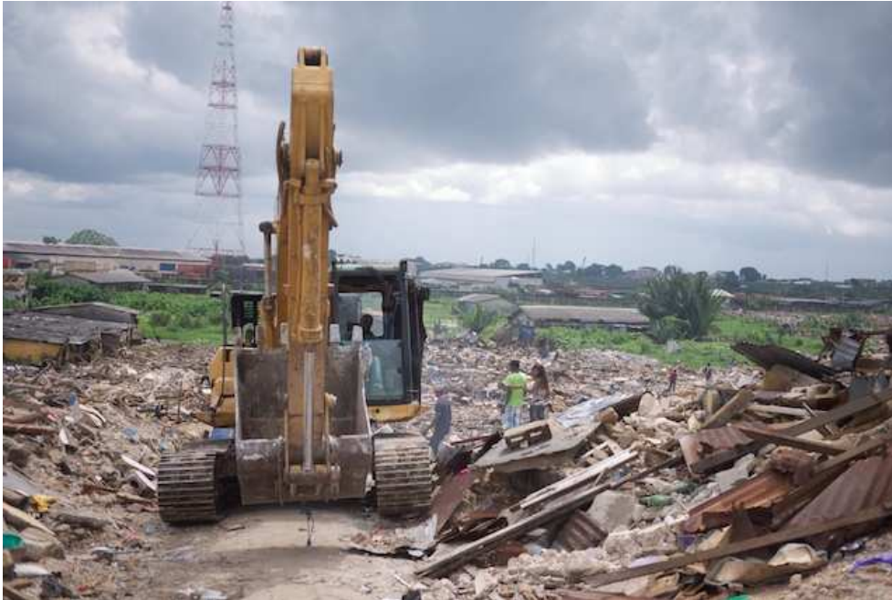
Women look as an excavator demolishes homes in Abonnema Wharf –Saturday 30 June 2012.
