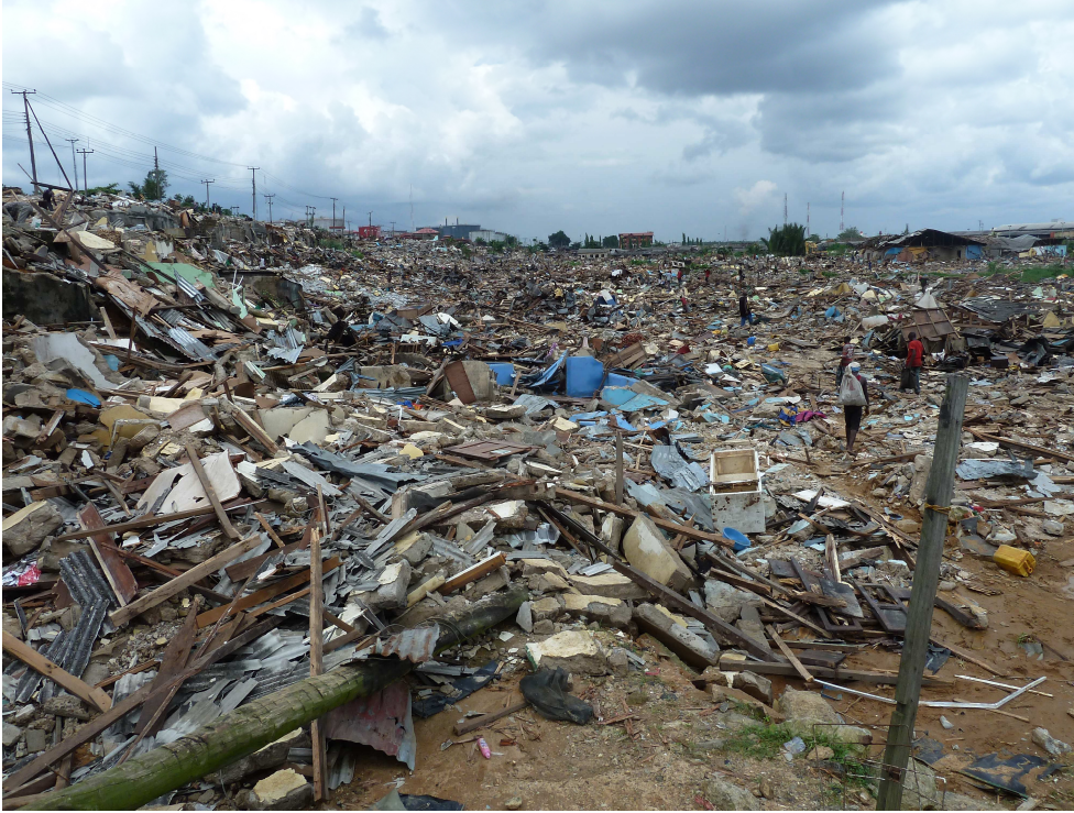
Abonnema Wharf, now a sea of rubble after five days of demolitions in the community - Sunday 1 July 2012.
