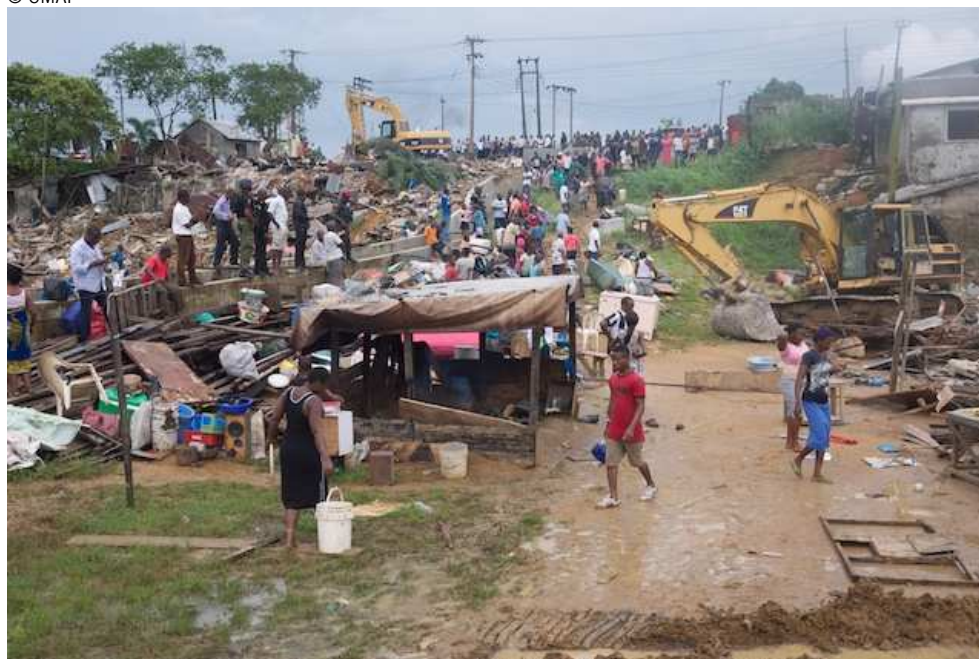
Wednesday 27 June 2012. Day one of demolitions in Abonnema Wharf, Residents look on at an excavator demolishing houses in the waterfront.
